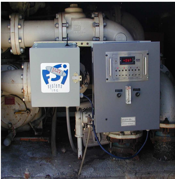
Phoenix Sentry Monitor installed at a wastewater lift station
